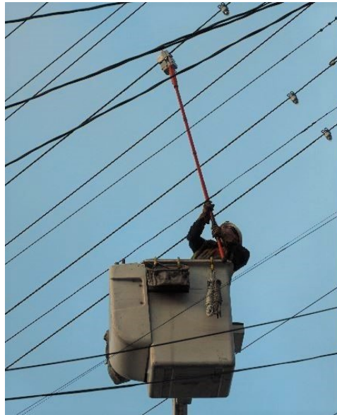
Figure 1: PG&E field test of Sentient Energy line sensors. Here line sensors are installed next to some of the 200,000+ mechanical FCIs PG&E has in place today. Line sensors are designed to replace these FCIs as a much more capable instrument.
